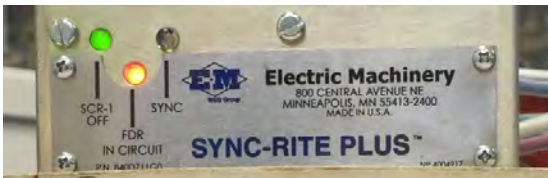
Resistors in Circuit and SCR-1 Attempting to Fire
